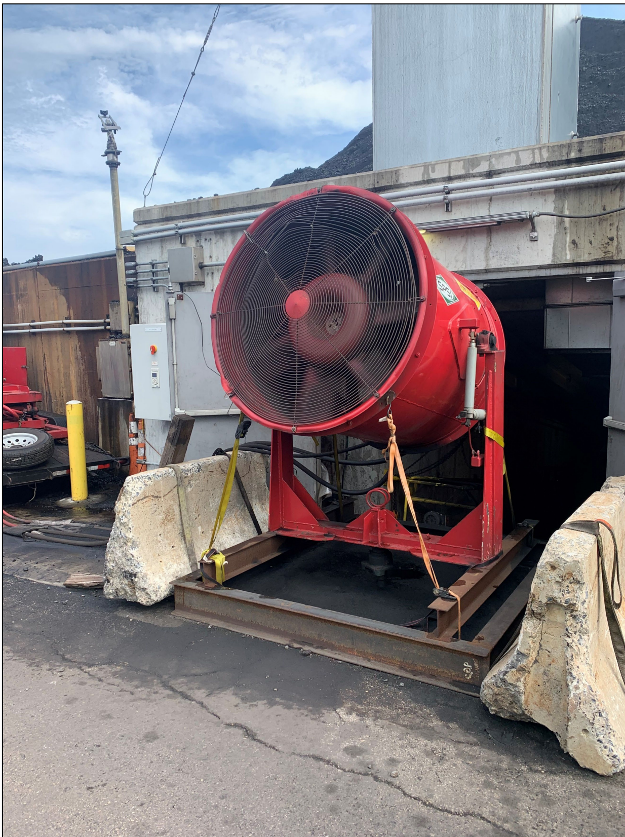
Figure 5.6.3. Temporary ventilation fan installed at south portal of South Reclaim Tunnel.
