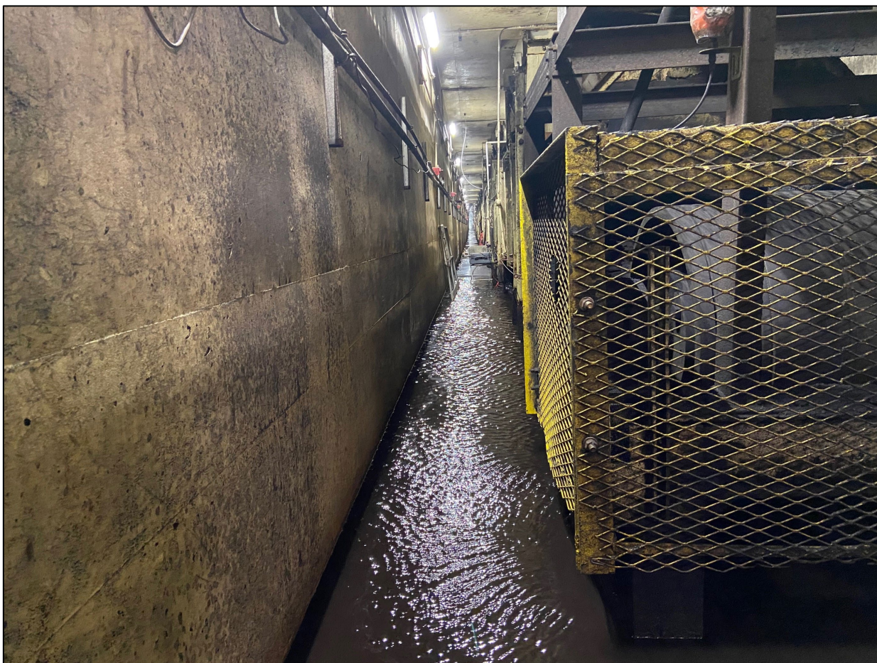
Figure 2.3.1. Washing walkways of South Reclaim Tunnel. View towards north from tail pulley enclosed in yellow grating.
