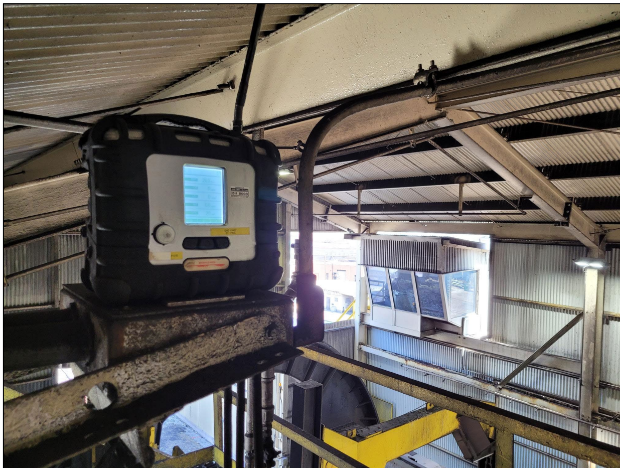
Figure 2.5.1. Air monitor in top level of railcar dumper shed. The yellow arm in the bottom of the picture is part of the counterweighted platform.
