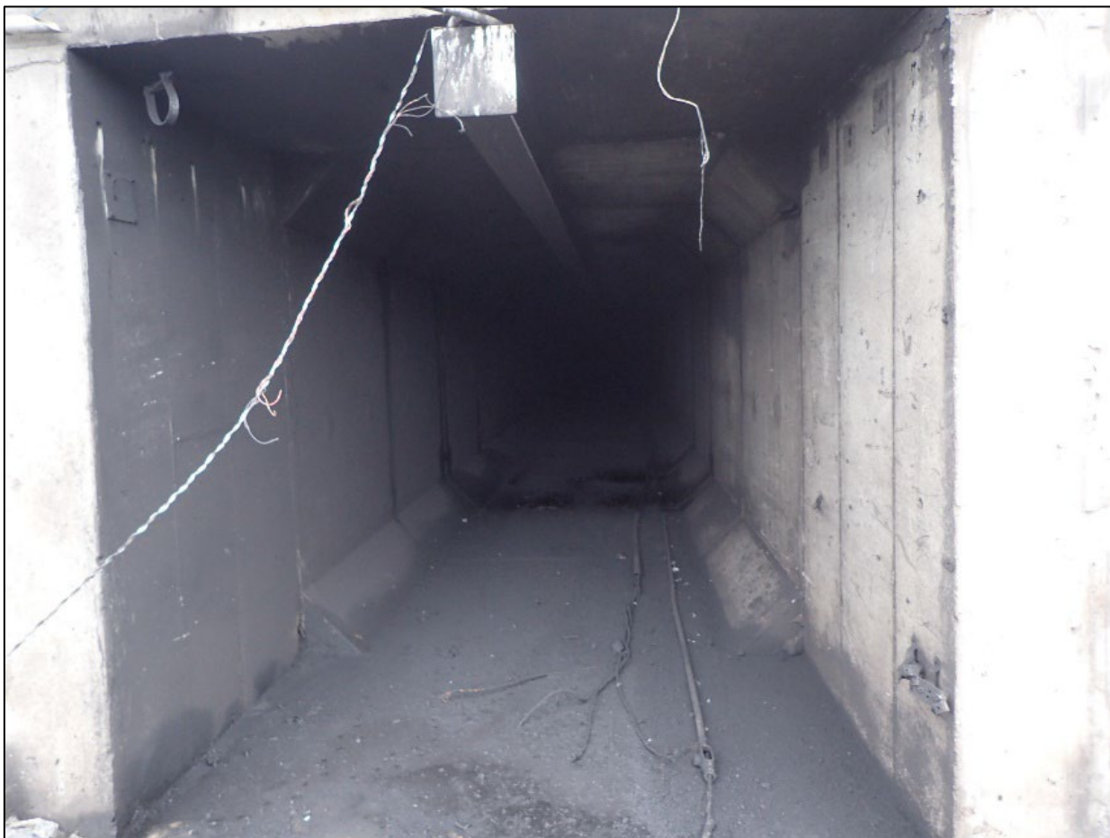
Figure 6.2.1. View east into escape tunnel portal. North wall (left in picture) is black; south wall is not.
