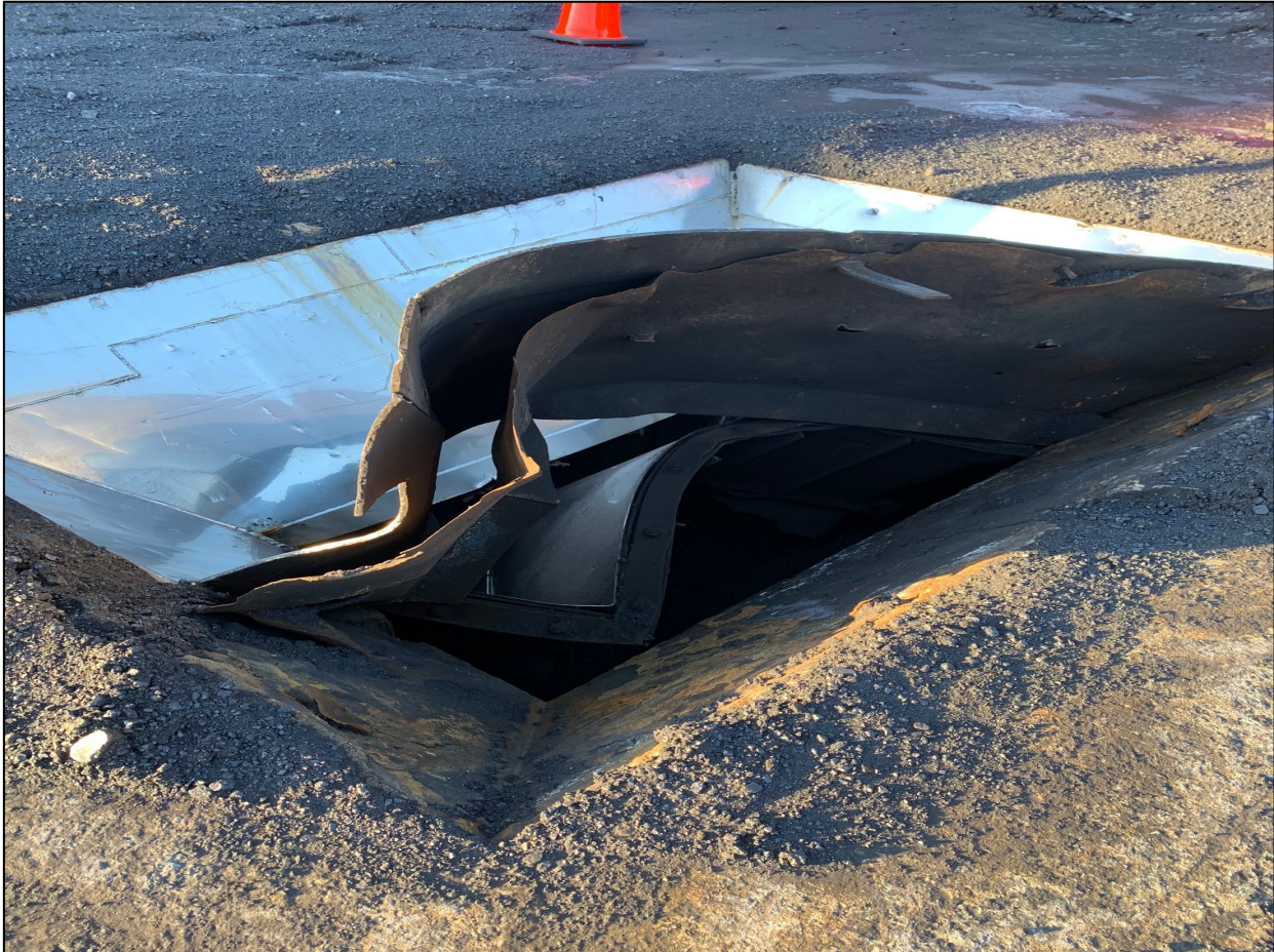
Figure 6.3.1. Feeder hole for VF-21 from the surface of the coal transfer yard.
