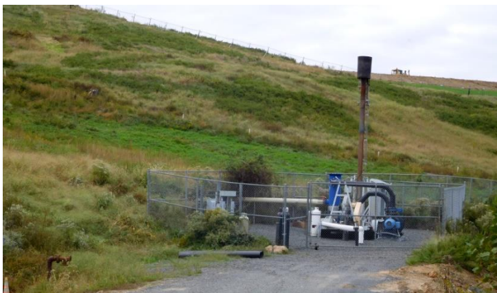
Over 1,100 municipal solid waste landfills reported emitting 3.3 million metric tons of methane to the Greenhouse Gas Reporting Program in 2021.
