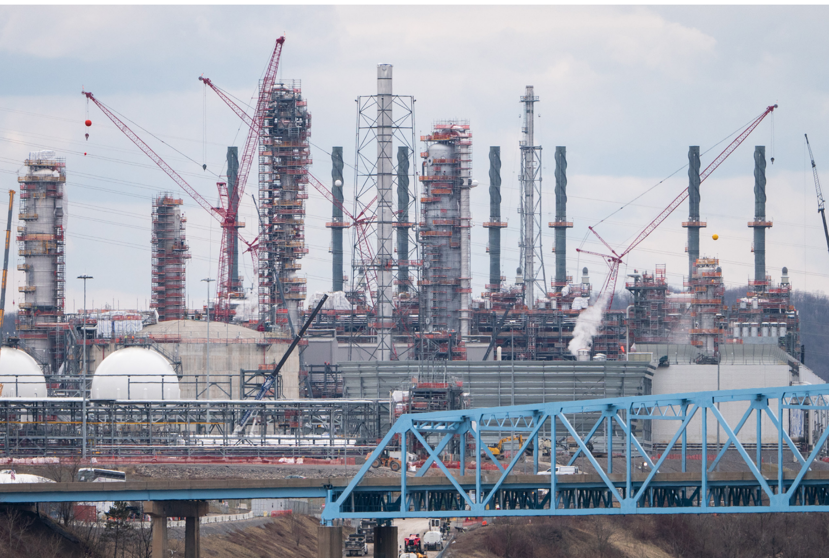
The Shell Monaca ethylene and plastics plant under construction northwest of Pittsburgh. Photo by Mark Dixon, Flickr.
