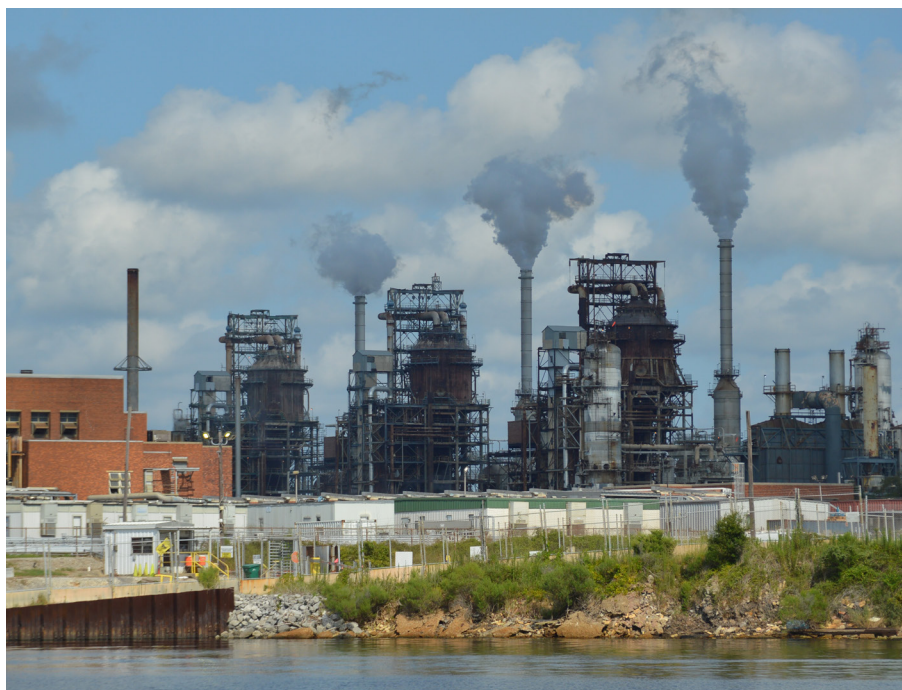
The largest boilers and heaters examined for this study were at the CITGO Lake Charles Refinery in Louisiana.
